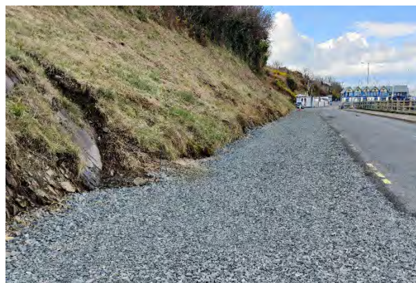
Fig. 2.03: The same location as in Fig. 2.02 (Site 2a) in April 2023 having been severely damaged. The seepage zone has been truncated and the small stream in the drainage channel has been entirely lost.
